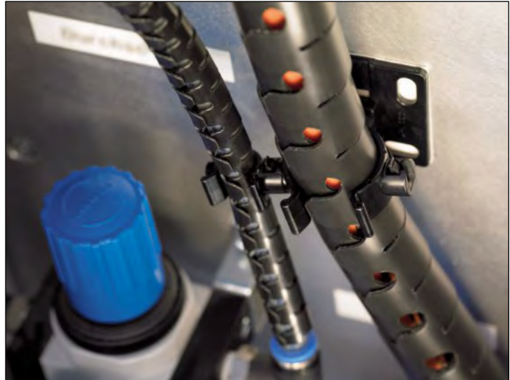
The protection and affixing of cables in a wiring cabinet with Helawrap sleeving.
